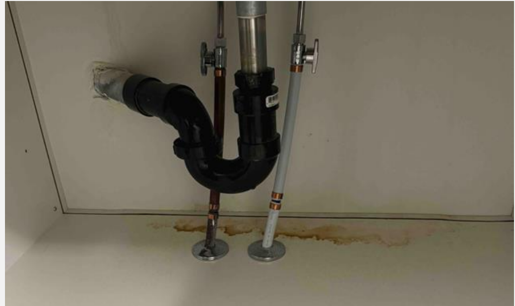
PHOTO F: Water damage in base cabinet floor
