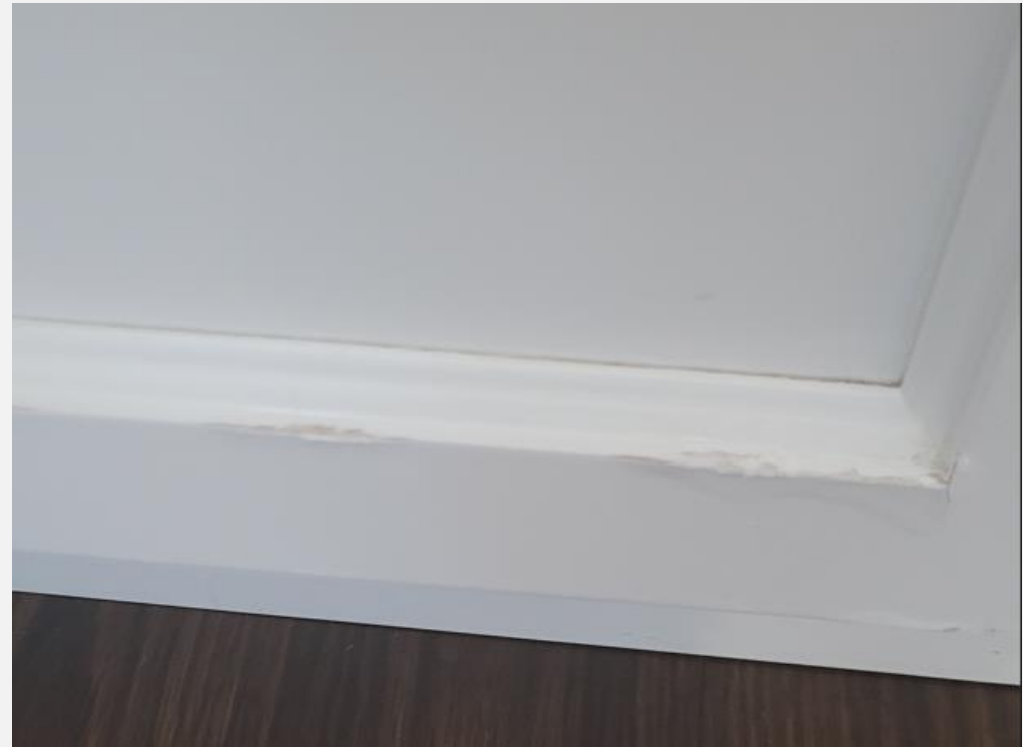
PHOTO H: Water saturation at lower base door.
