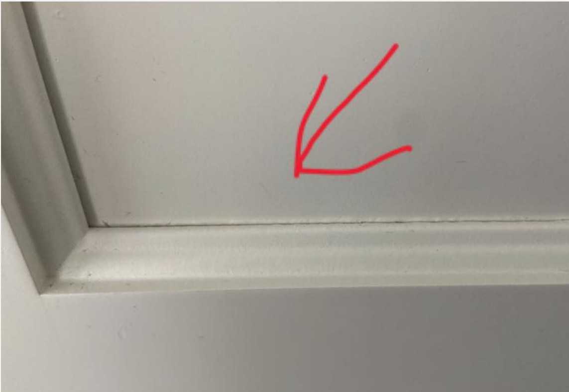
PHOTO E: Cracks/bubbling caused by water permeation
